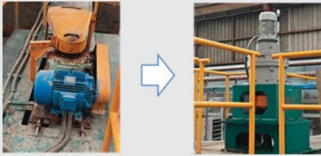
Project to reduce the agitator motor from 11 kW to 4 kW
